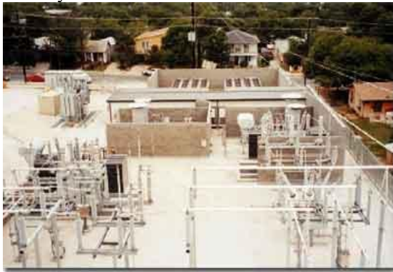
Figure 4.3 over view of Eagle Pass VSC - HVDC station [16]
